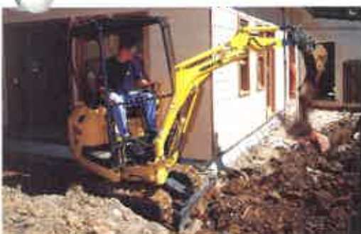
Omega Plumbing's Komatsu PC12-8 is able to work in very confined spaces.
