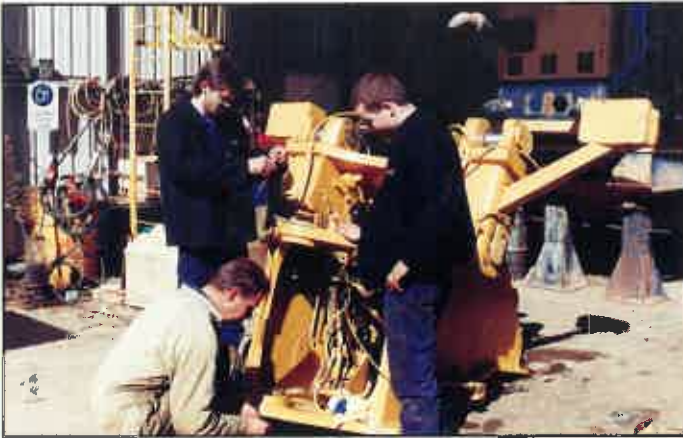
Lyal Hooper, Craig Wojtowicz and Peter Gorrie measure a WA380 front frame.
