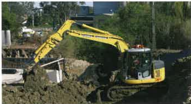
W&D Elliott's newly purchased PC138US-2 excavator gives more versatility in confined space work.
