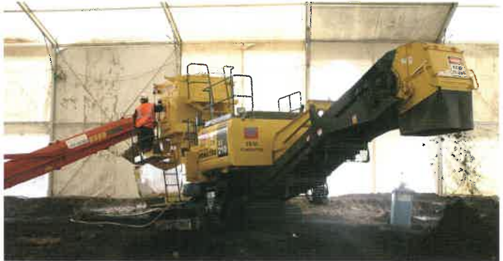
EESI Contracting's BZ210 Reterra soil recycler working on a former gasworks site in Melbourne. It works entirely within a pressurised tent structure to minimise unpleasant odours affecting the surrounding area.
