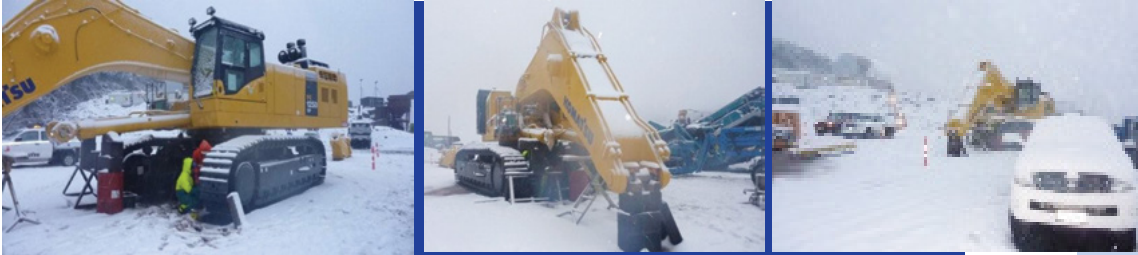
Komatsu NZ assembled and commissioned the PC1250SP-8 excavator under extreme weather conditions
