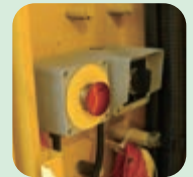
Engine room rear
