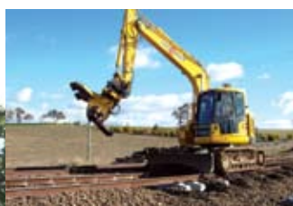
In addition to the rubber tracks, the excavators have also had hydraulic modifications to take Engcon rotating hitches, giving the ability to tilt and rotate 360°, to increase the ease of the side insertion process.
