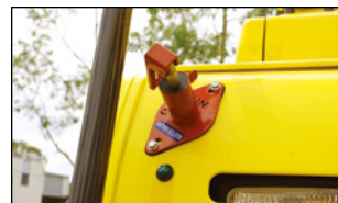
Battery Isolation Single pole, lockable Bosch-type battery isolation.
