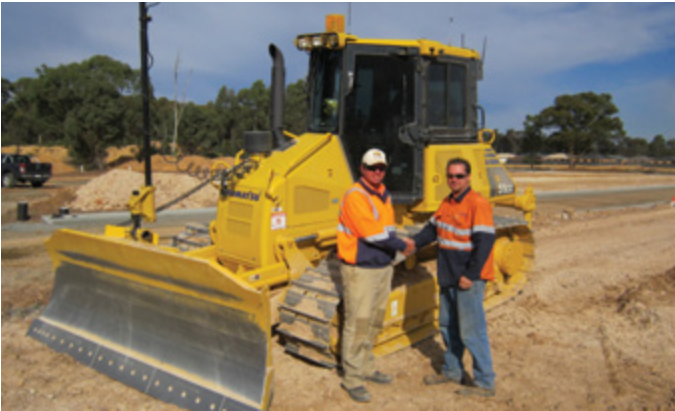
Left: Ash Beriman-Mckinnon Earthmoving & Shane OBrien, victorian Machine Control Support/Install for Position Partner.
